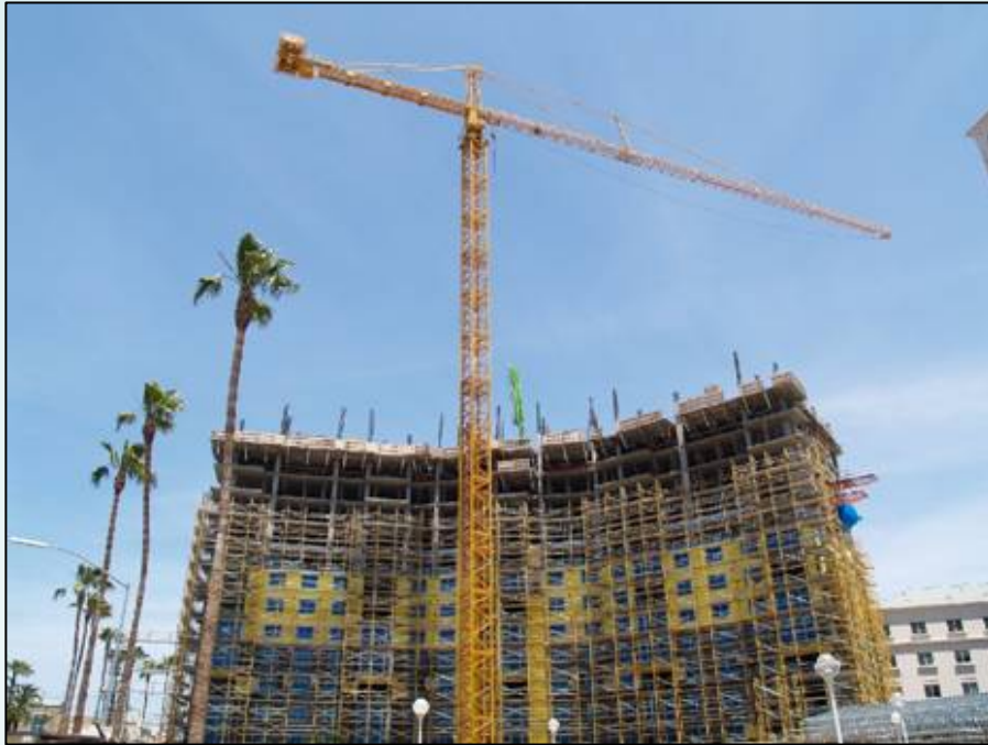
Hammerhead Type Tower Crane
